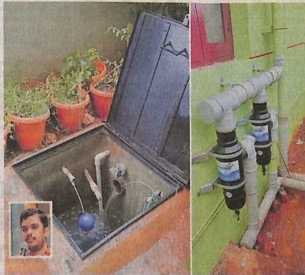
Rainwater harvesting calls for pipes, filters and a sump. Since 2019, Ganesh (inset) has helped about 150 apartment complexes set up RWH systems in Bengaluru.
